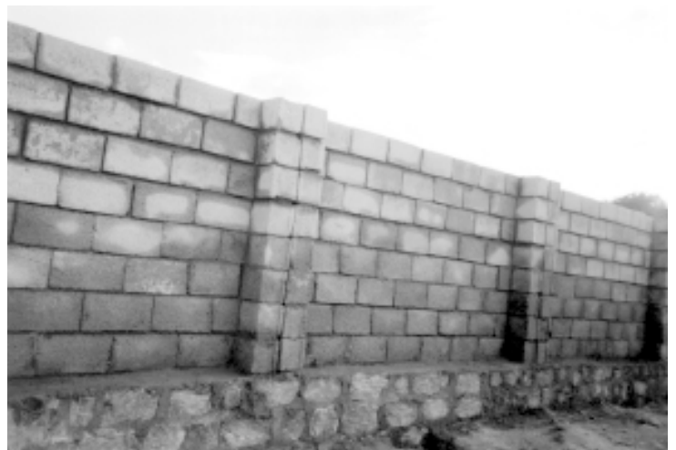
October, 1998. A part of the raising wall is seen. Two sides of the wall is completed. Western and Southern side walls are constructed fully.
