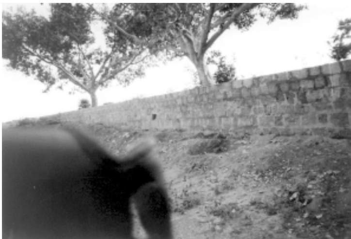
September, 1998. Eastern side foundation wall is seen. Land area is hidden. The trees seen are the project land.
